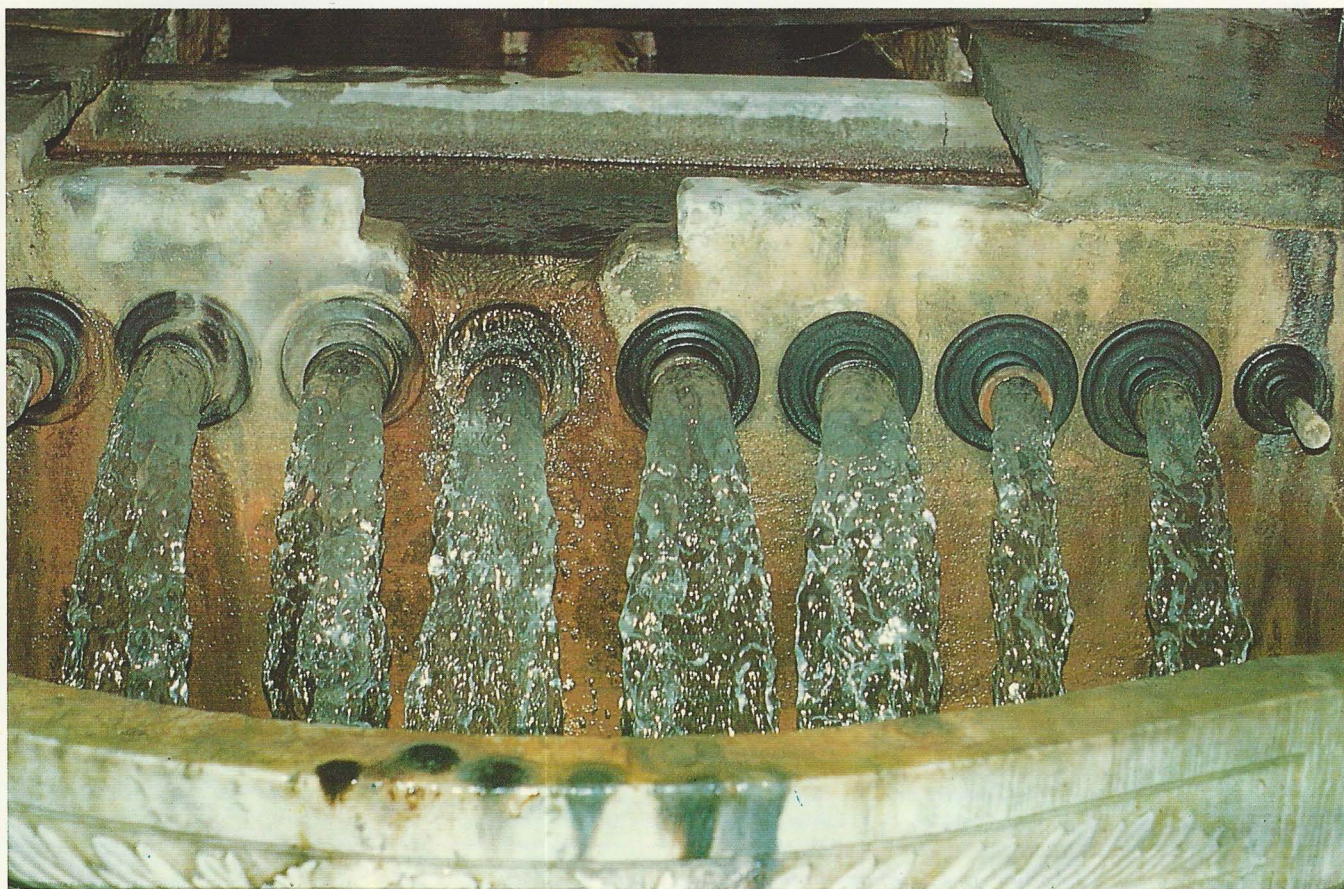
Discharge measuring system at Sultan Mahmud Dam
